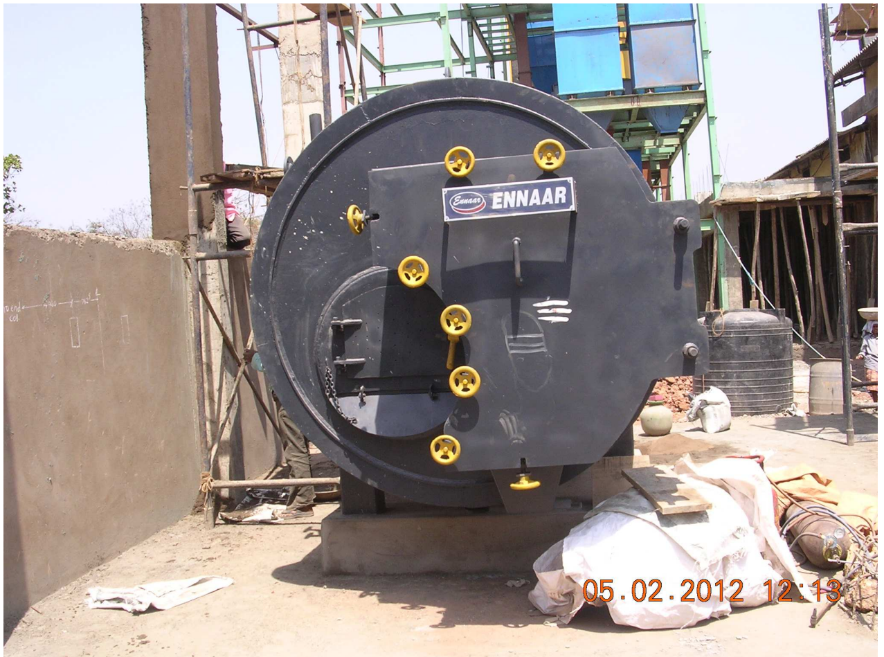
1.0 Ton wood fire boiler
